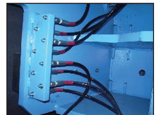
2 Centralized greasing point
